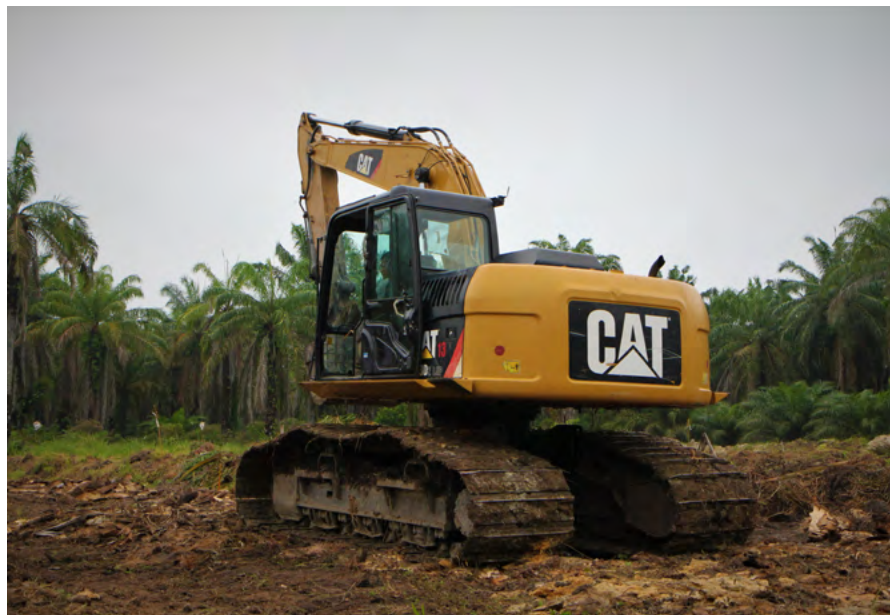
Best management practices for replanting include using an excavator for felling and trunks to be cut into manageable size by chain saws.
